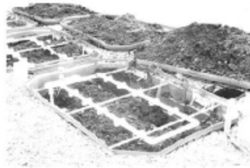
Peat Filter With Distribution Manifolds Source: Performance Evaluation of a Recirculating Sand Filter and Peat Filter in West Virginia, Small Flows Quarterly , Winter 2003, Volume 4, Number 1.
